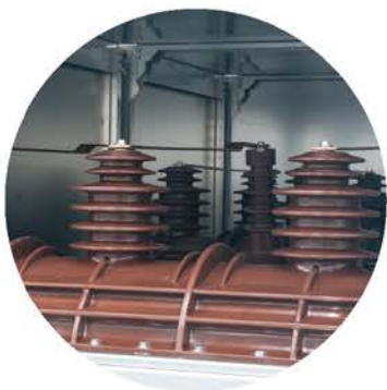
MAIN BUSBAR SECTION
